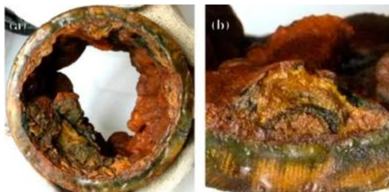
Figure 9: Heavily corroded internal surface of cast iron pipe used in drinking water distribution systems. (a) Pipe cross section, (b) tubercle. Credit: Mi et al., 2015
